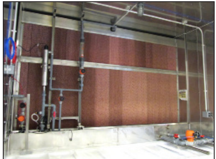
Evaporative Cooler Air Leaving Side
