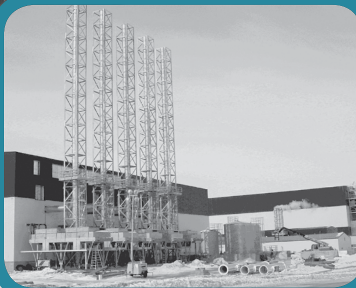
Generator & Fume Exhaust
