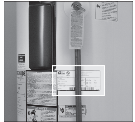
The water heater’s electrical requirements can be determined from the data plate.
