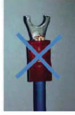
Terminal has been cut.
