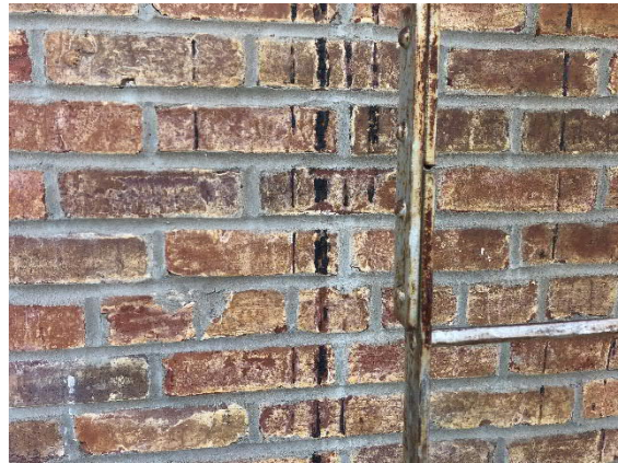
Photo #10 Remnant roofing tar observed on the wall.
