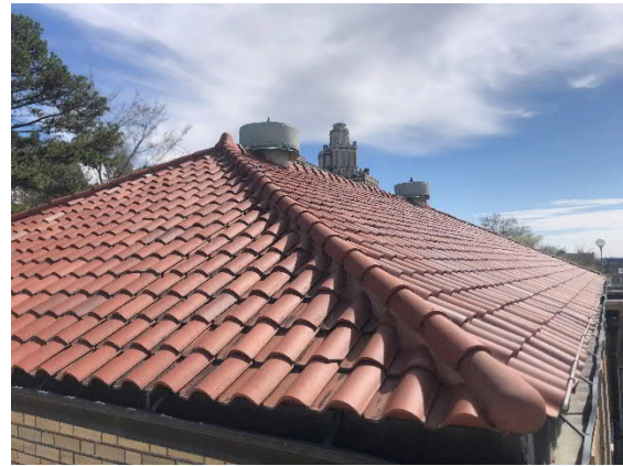
Photo #4 Terracotta shingles.
