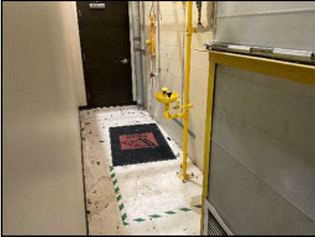
35 - B202 Eyewash Station Obscured by Screen Wall
