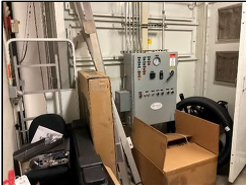
46 - B202 Paint Booth
