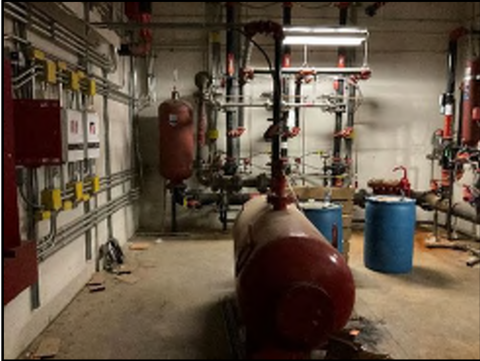
37 - B202 Fire Riser Room #1
