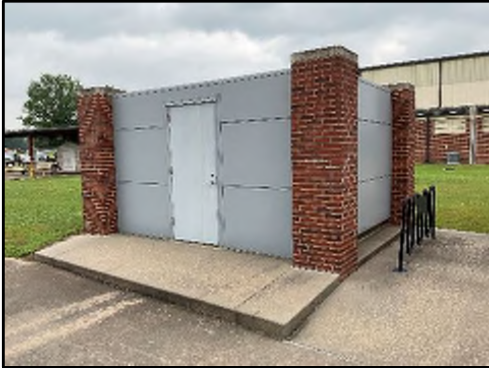
27 - B202 Transformer Enclosure
