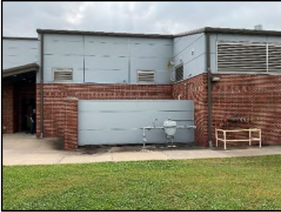
51 - B202 Utility Enclosure
