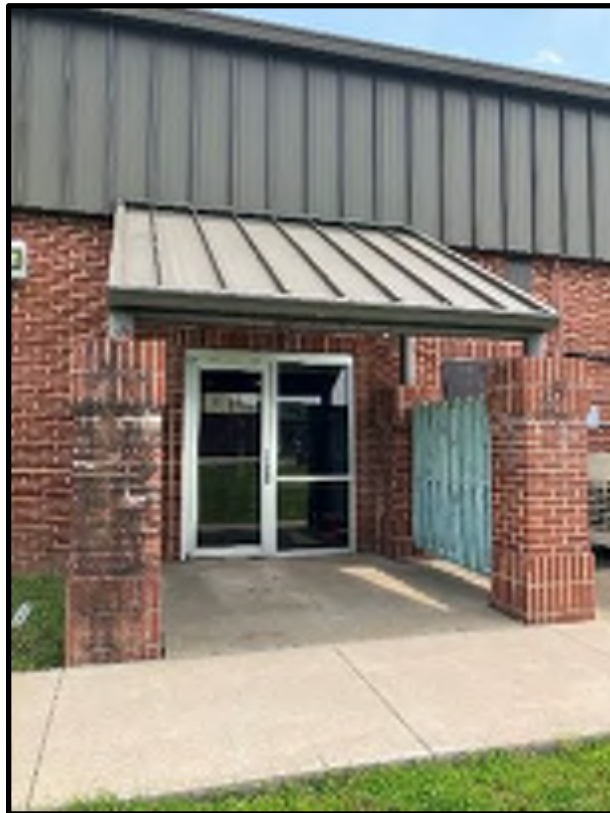
4 - B201 Covered Entry Brick Deterioration
