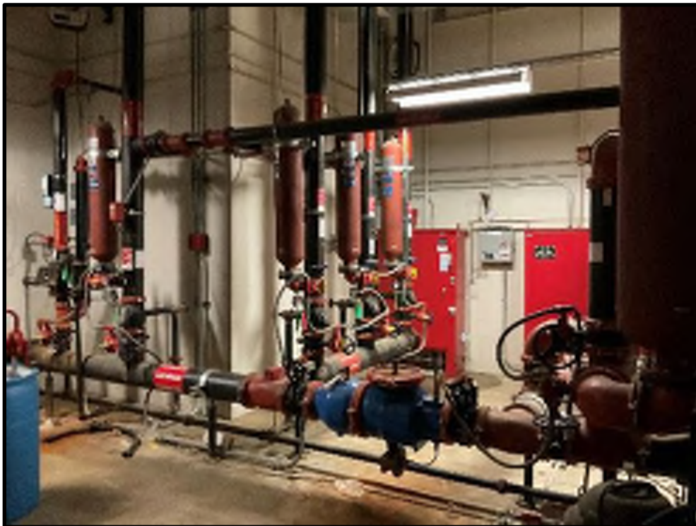
38 - B202 Fire Riser Room #2
