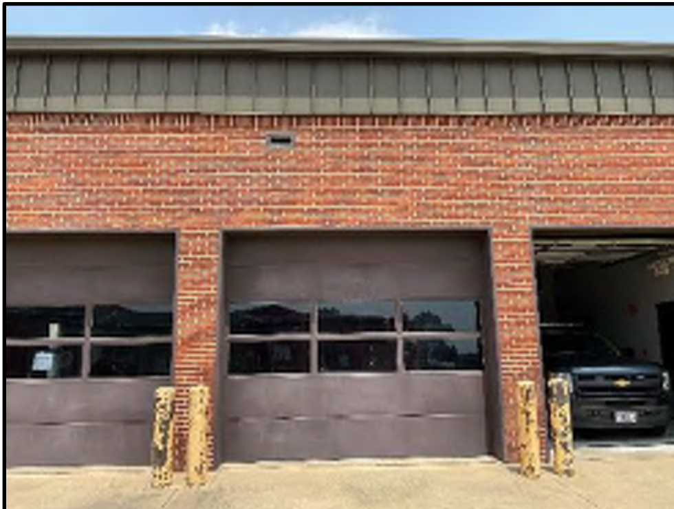
6 - B201 Infill South Doors
