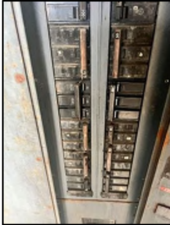
63 - B214 Old Electrical Panel
