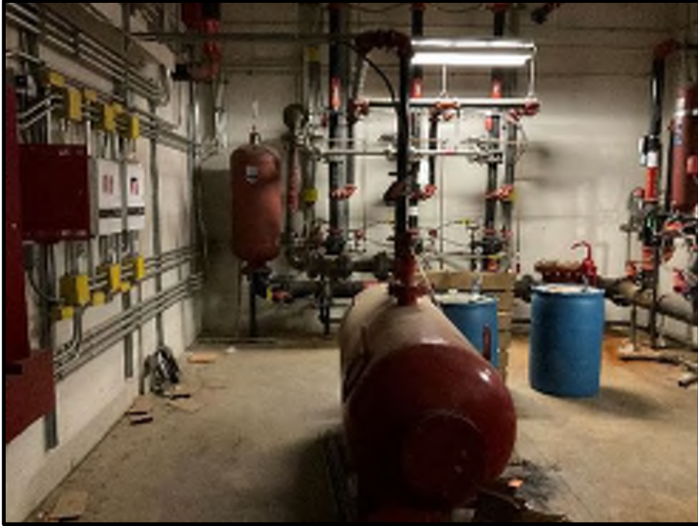
37 - B202 Fire Riser Room #1
