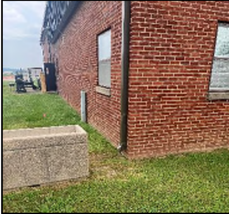
9 - B201 Downspout with No Splash Block
