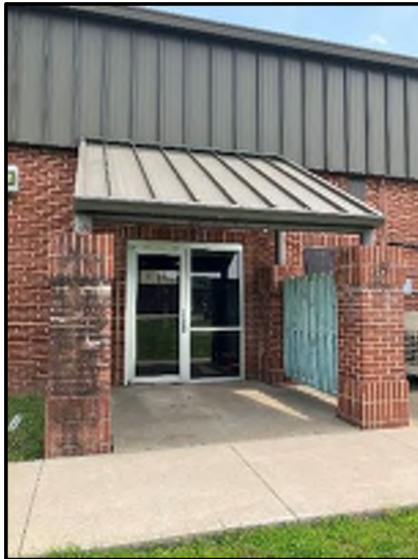
4 - B201 Covered Entry Brick Deterioration
