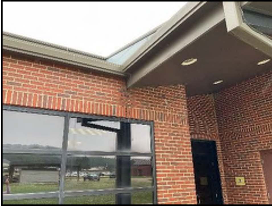
21 - B202 Water Damage at Covered Entry
