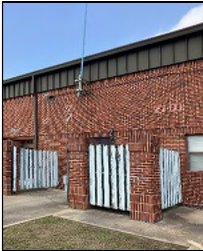
8 - B201 Utility Enclosure #2
