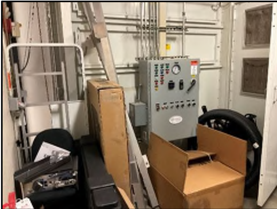
46 - B202 Paint Booth
