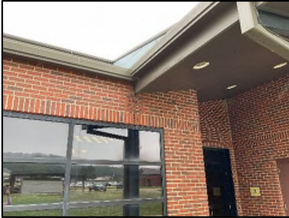
21 - B202 Water Damage at Covered Entry
