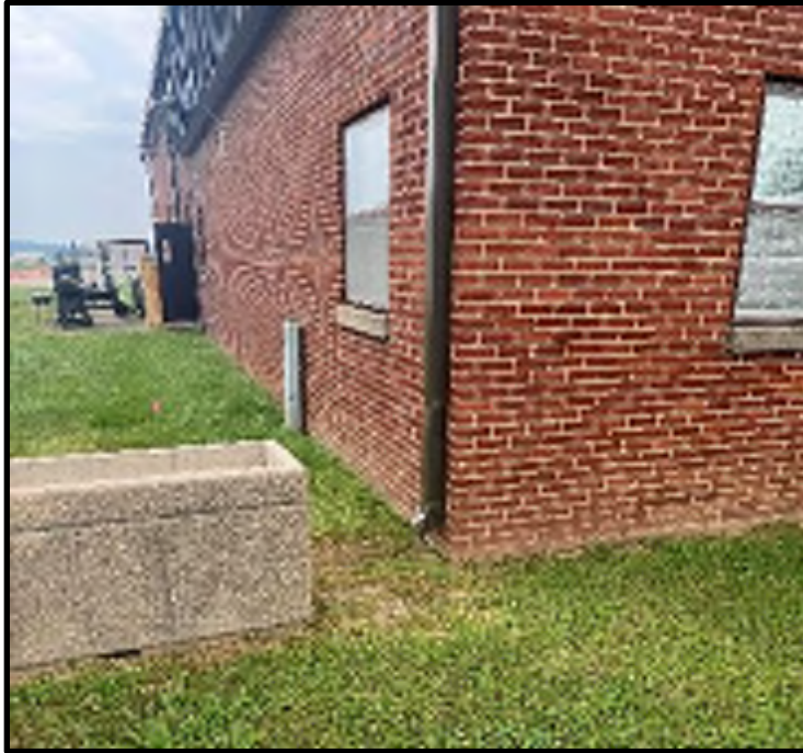
9 - B201 Downspout with No Splash Block
