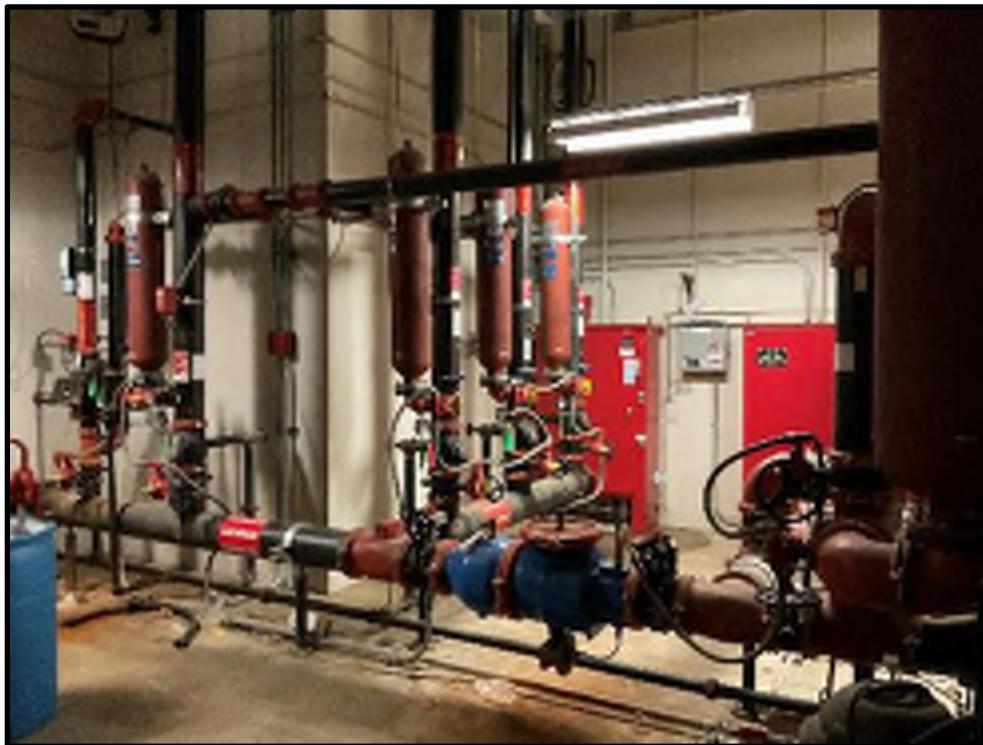
38 - B202 Fire Riser Room #2
