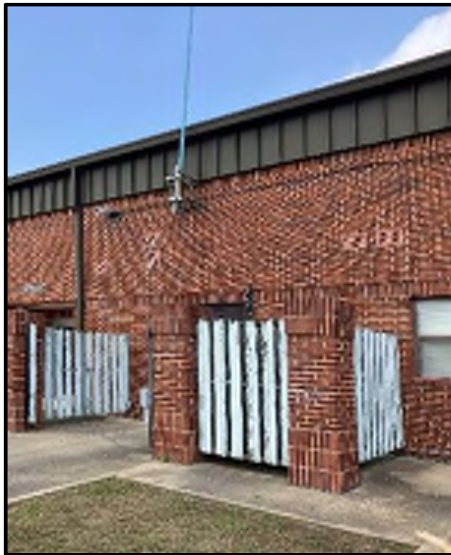
8 - B201 Utility Enclosure #2
