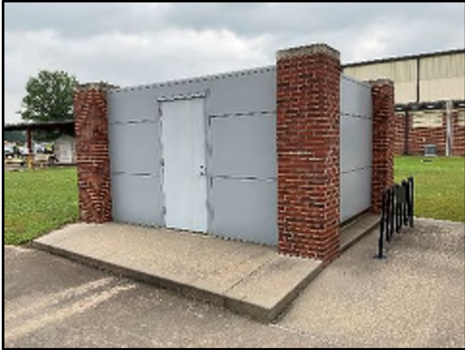
27 - B202 Transformer Enclosure
