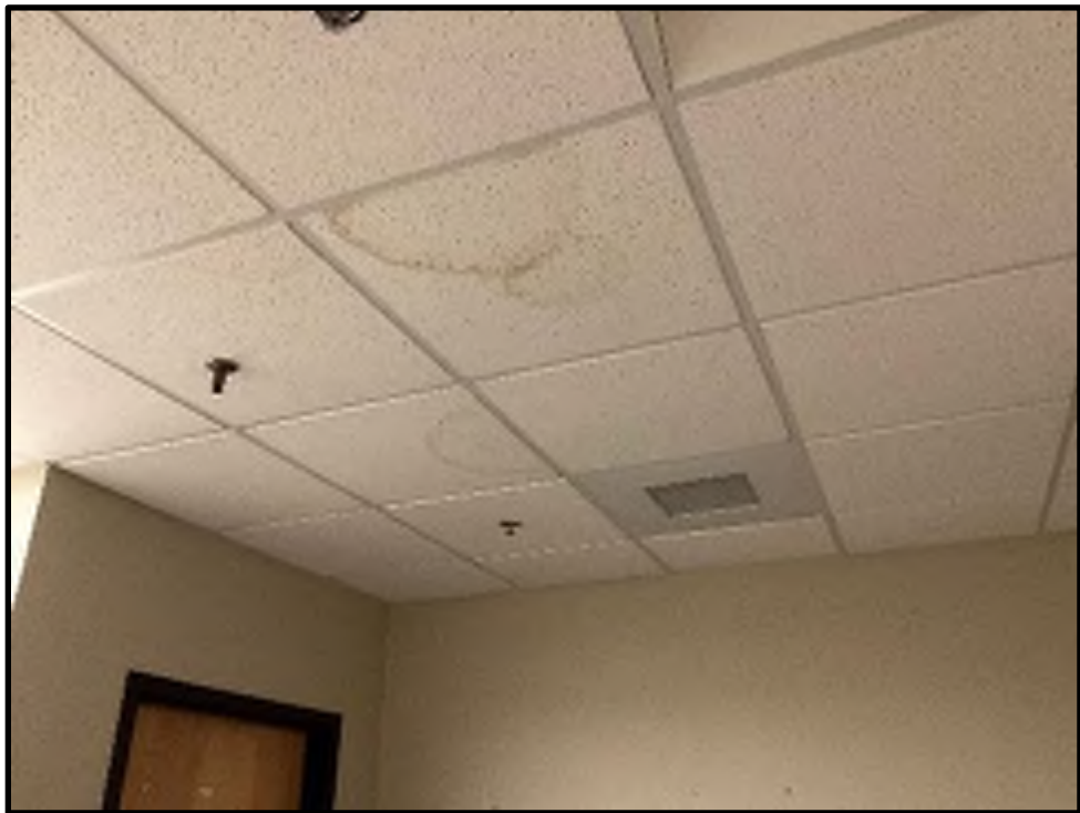
30 - B202 Example of ACT Damage
