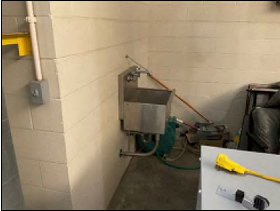
45 - B202 Hangar Bay 3 Tyre Sink
