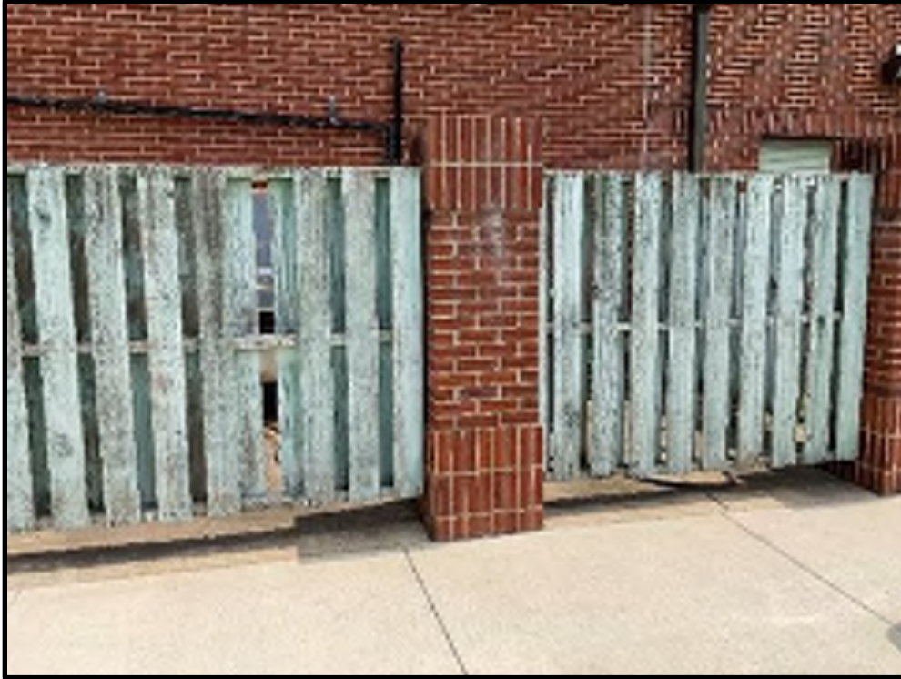
7 - B201 Utility Enclosure #1
