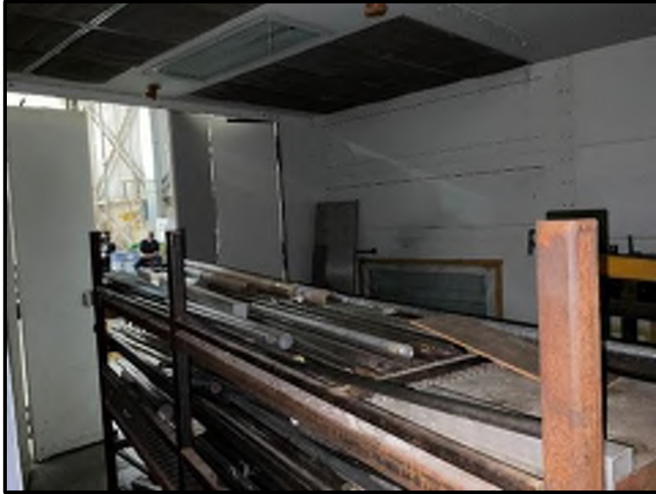
47 - B202 Paint Booth Interior
