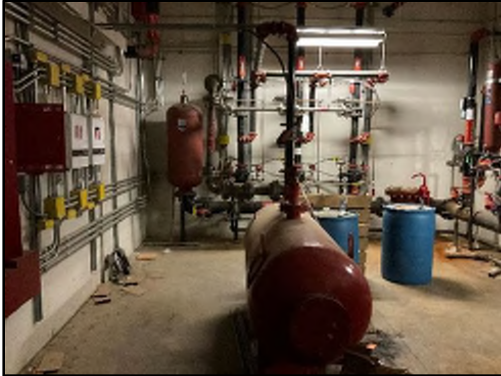
37 - B202 Fire Riser Room #1
