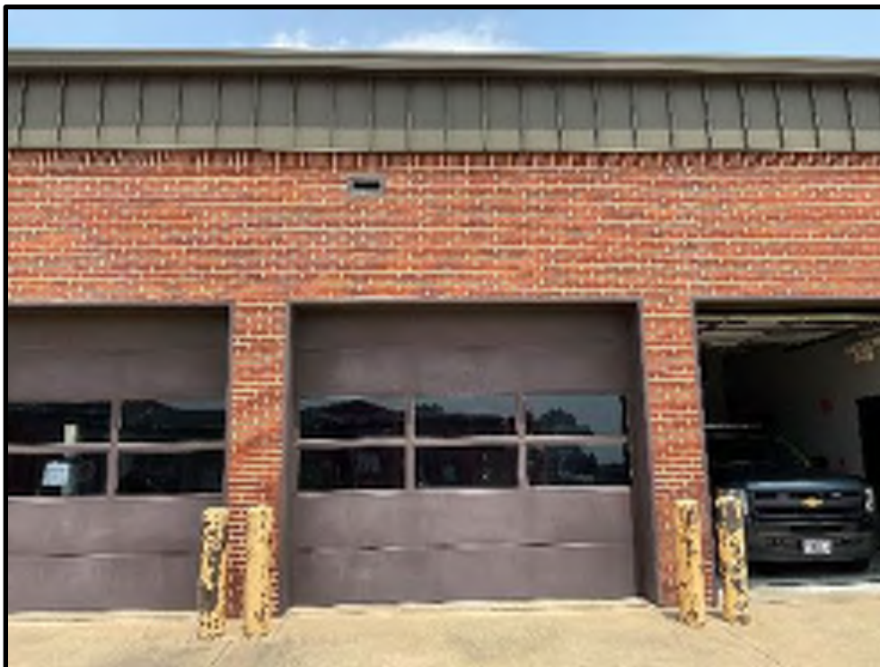
6 - B201 Infill South Doors
