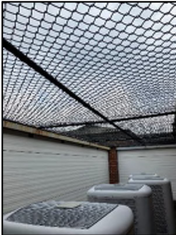
50 - B202 Utility Enclosure
