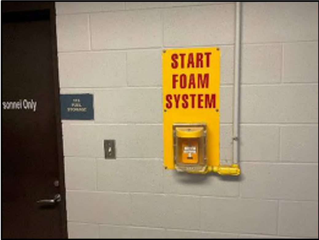
54 - B202 Foam Suppression System
