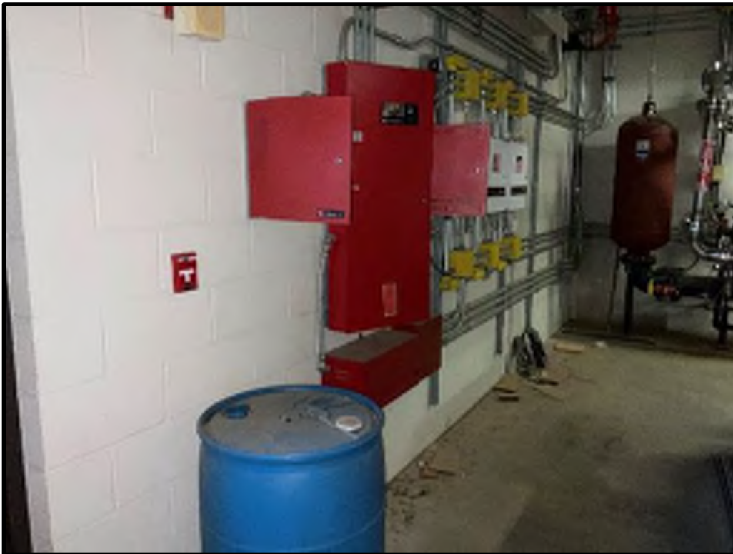
36 - B202 Fire Riser Equipment
