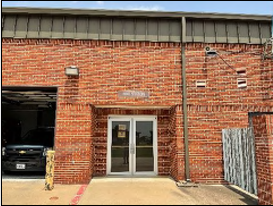
11 - B201 Infill South Doors
