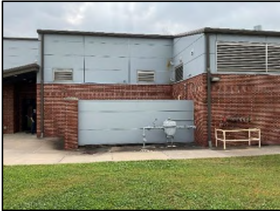
51 - B202 Utility Enclosure
