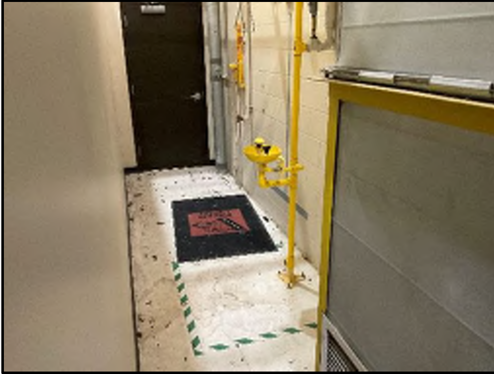
35 - B202 Eyewash Station Obscured by Screen Wall
