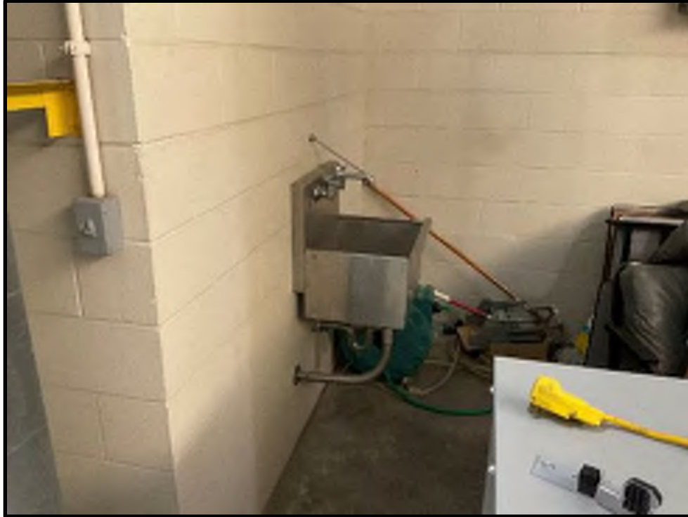
45 - B202 Hangar Bay 3 Tyre Sink
