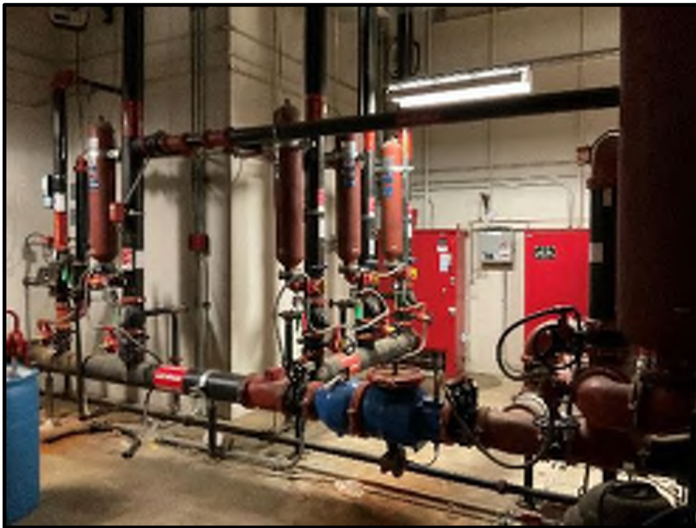
38 - B202 Fire Riser Room #2
