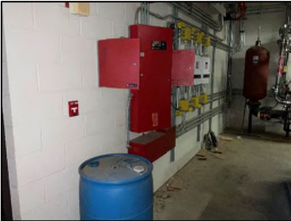
36 - B202 Fire Riser Equipment
