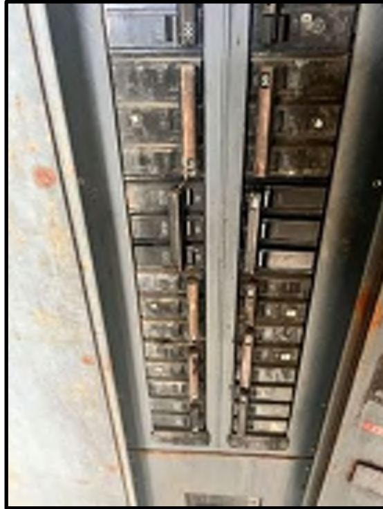
63 - B214 Old Electrical Panel
