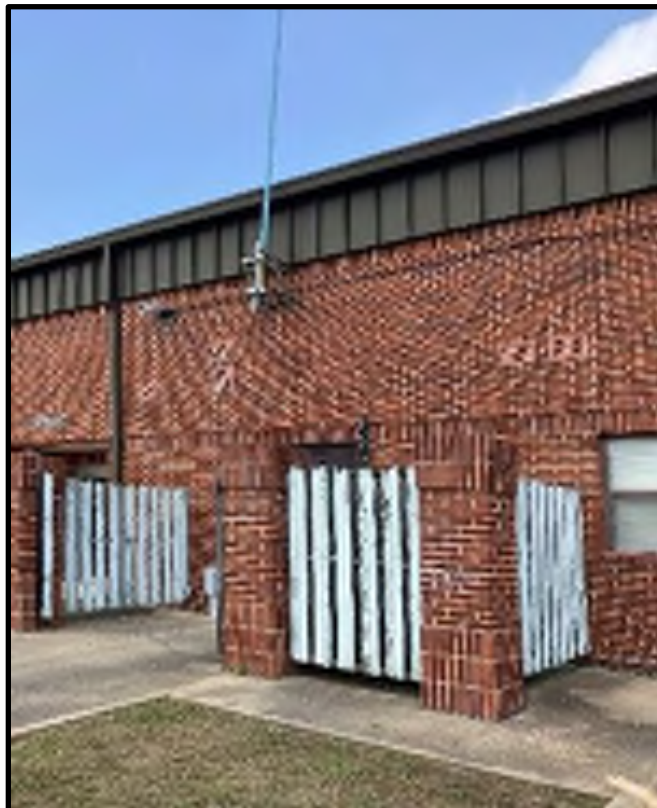
8 - B201 Utility Enclosure #2
