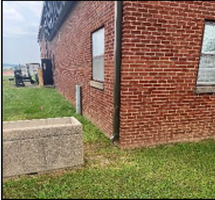
9 - B201 Downspout with No Splash Block
