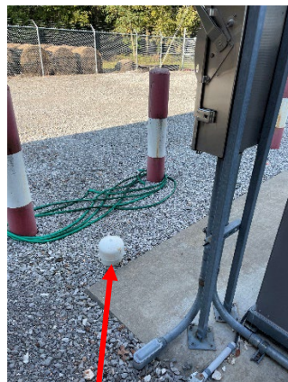
Figure 24: When new pad is installed locate new HVAC unit away from this cleanout.
