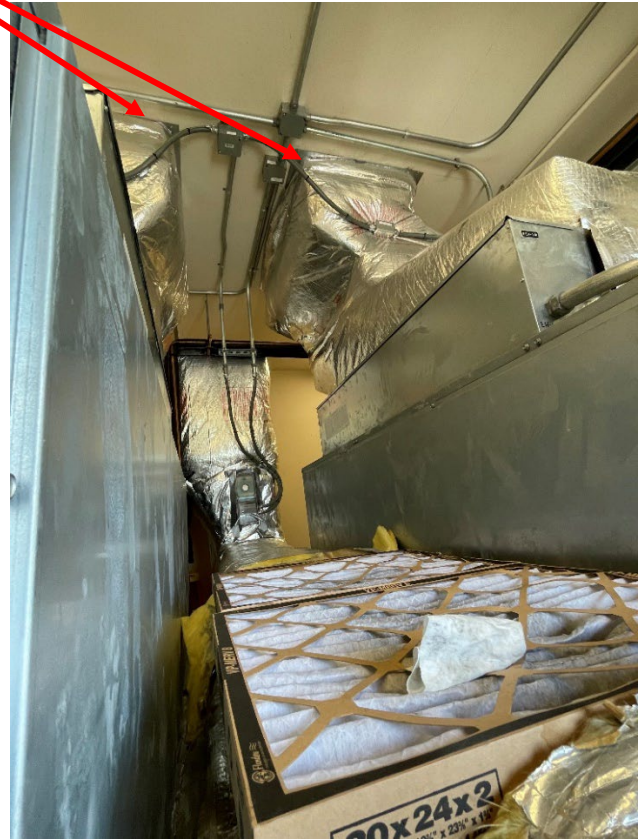
Figure 15: Location where new supply duct will connect to existing supply duct. Blank cover opening on the one to left.
