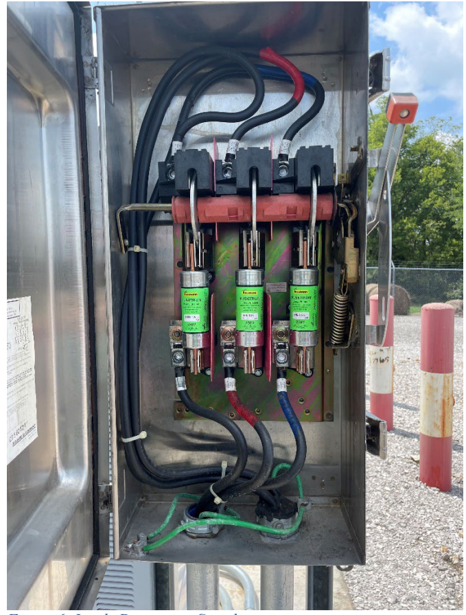
Figure 6: Inside Disconnect Switch
