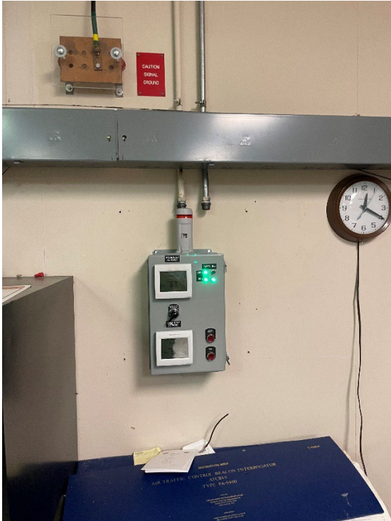
Figure 11: Existing HVAC Thermostats/Controls (To be Reused)
