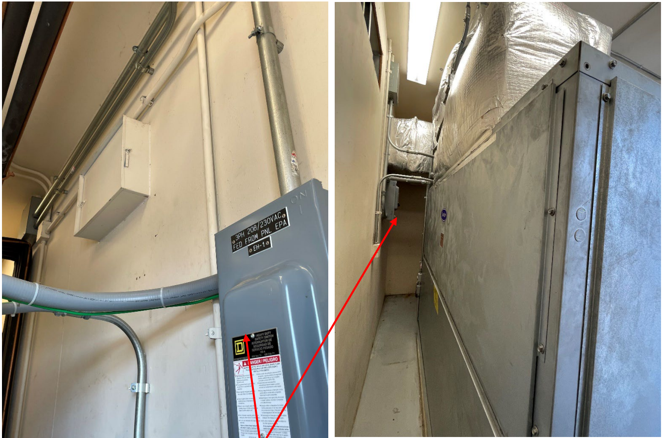
Figure 19: Remove Duct Heater Disconnect Switches
