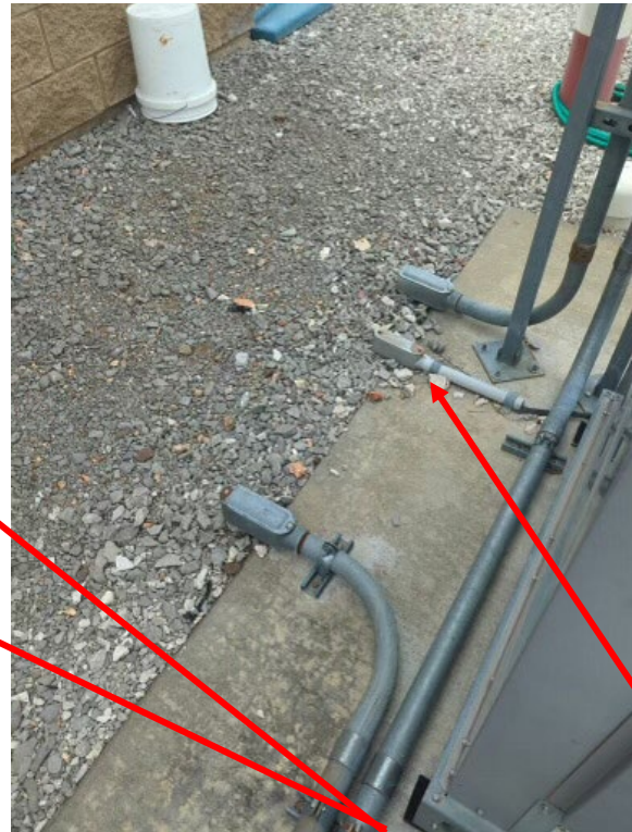
Figure 7: LBs showing Power Feeds to Unit Disconnects and PVC LB for Ground Wire
