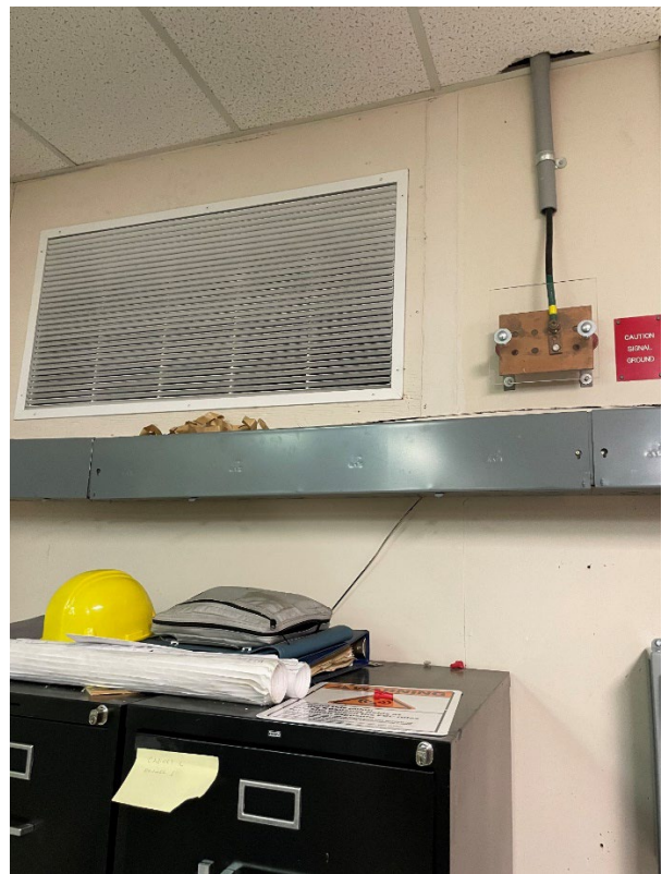
Figure 10: Existing Return Air Grille Close to Ceiling. Patch Hole and Refinish Drywall
