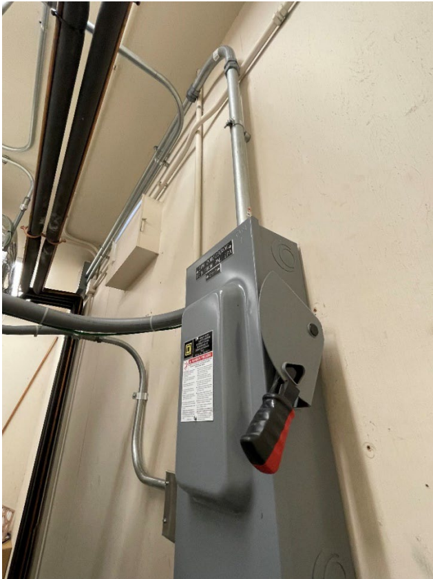
Figure 14: Interior Disconnect Switch for Duct Heater (Typ 2) to be removed.
