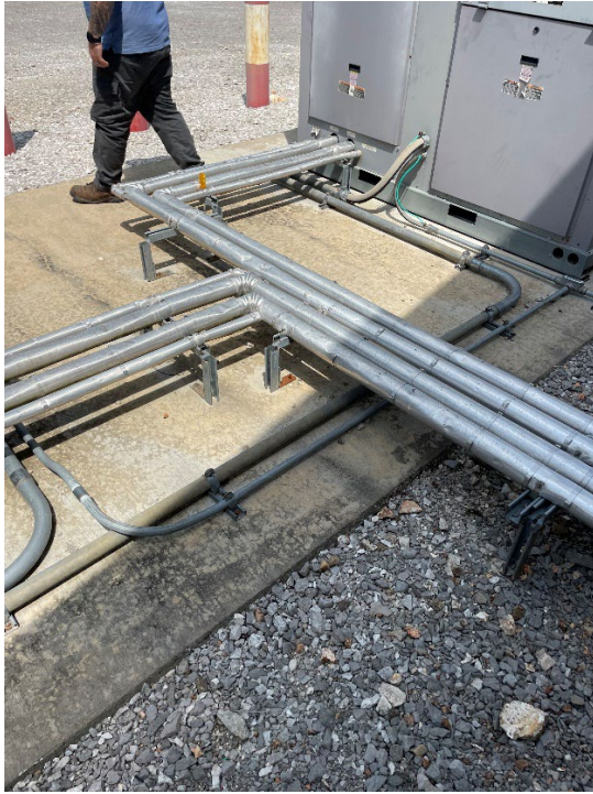
Figure 8: Refrigerant Lines (To Be Removed) Control conduit visible in photo. (3/4" RGS)
